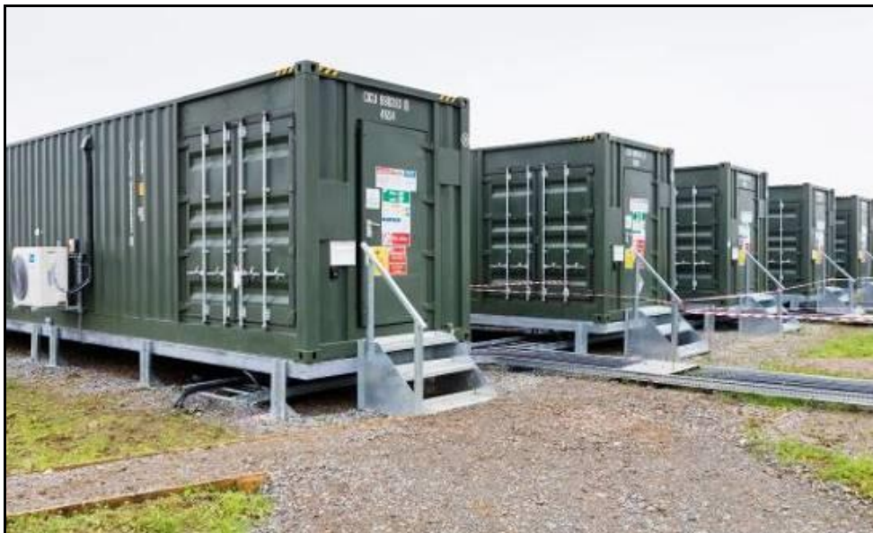
Photograph 1.2: Example of BESS located in storage containers
