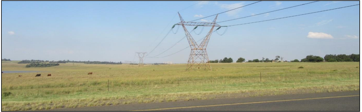
Photograph 3.11: 400 kV line traversing N11 approximately 6 km south of Ermelo
