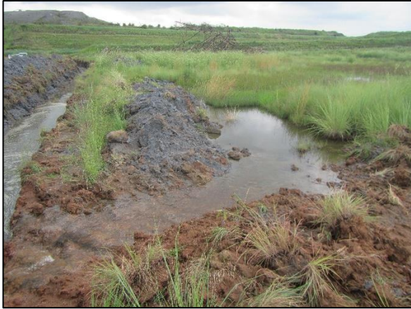
Figure 18: Drainage channels that have been excavated by power station management to prevent the flooding of access roads.
