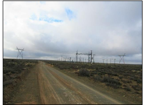
Figure 11: 22kV power lines and associated substation south of the Koup 1 WEF application site, adjacent to the N12.
