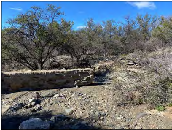
Figure 19: Several small weirs were found within the steeper valleys through-out the study area, most no longer functional
