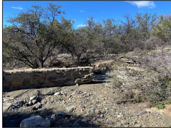
Figure 20: Several small weirs were found within the steeper valleys through-out the study area, most no longer functional
