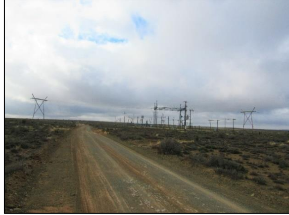
Figure 11: 22kV power lines and associated substation south of the Koup 1 WEF application site, adjacent to the N12.
