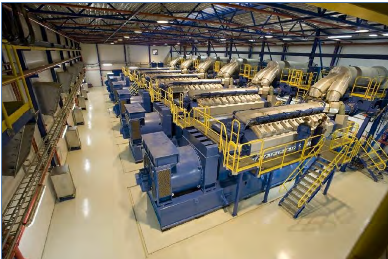
Figure 2-6: Interior of a typical gas engine power plant (Wärtsilä, Finland)
