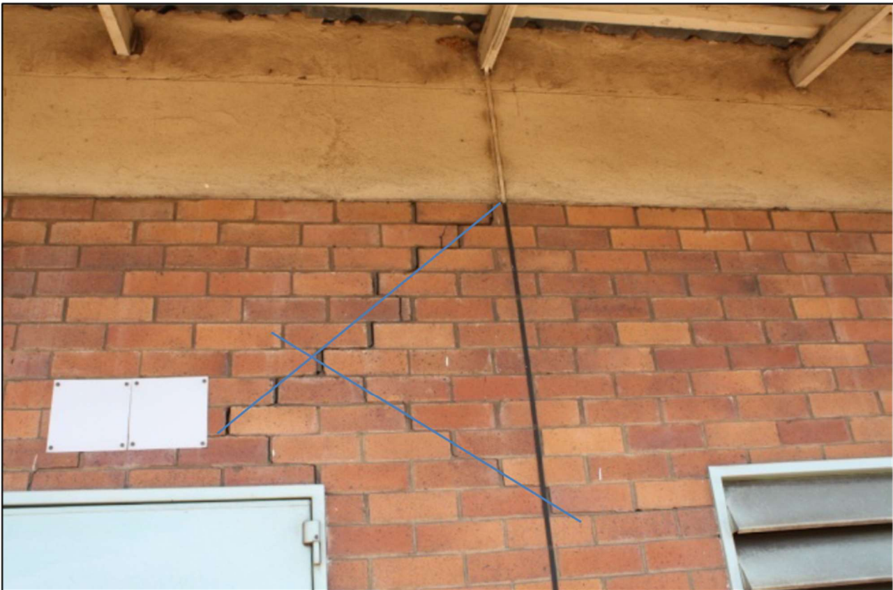
Figure 7: Example of blast induced damage.
