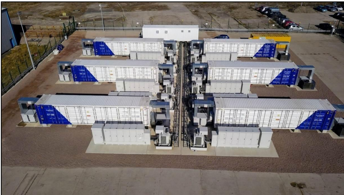
Photograph 1.2: Example of BESS located in storage containers
