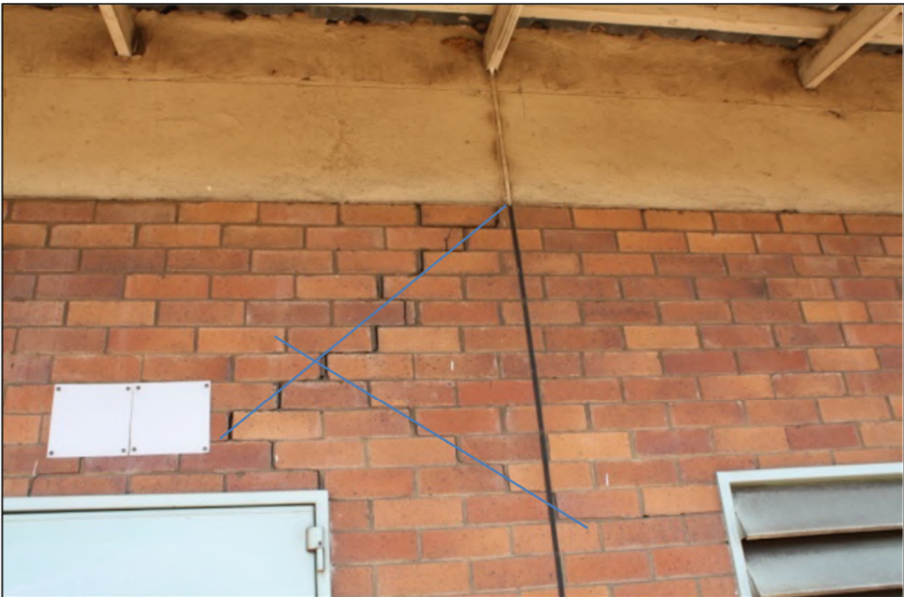
Figure 6: Example of blast induced damage.
