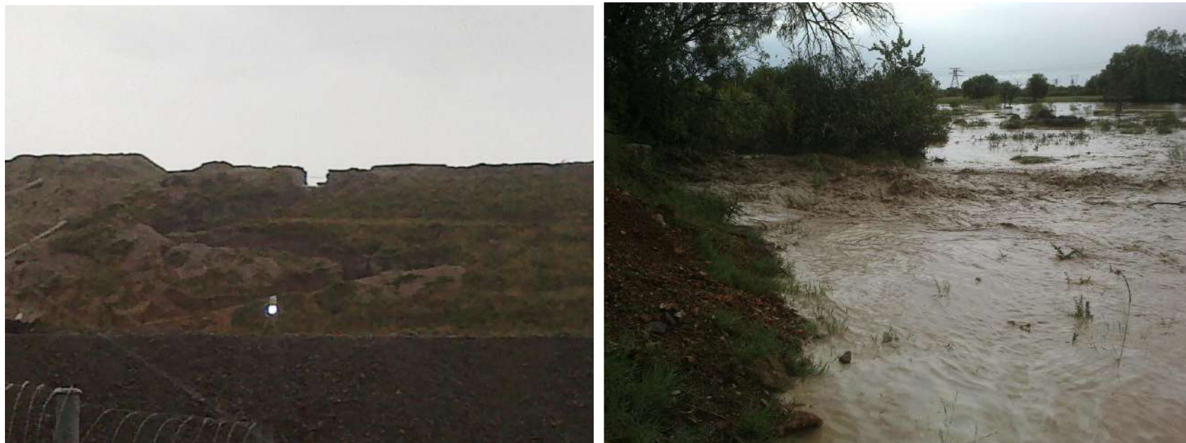
Failure of Tailings Storage Facility's walls with resultant spillages of toxic and radioactive slurry on farmland and into the Koekemoerspruit
