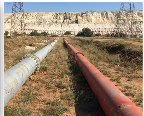
Secondary Containment Bunds
