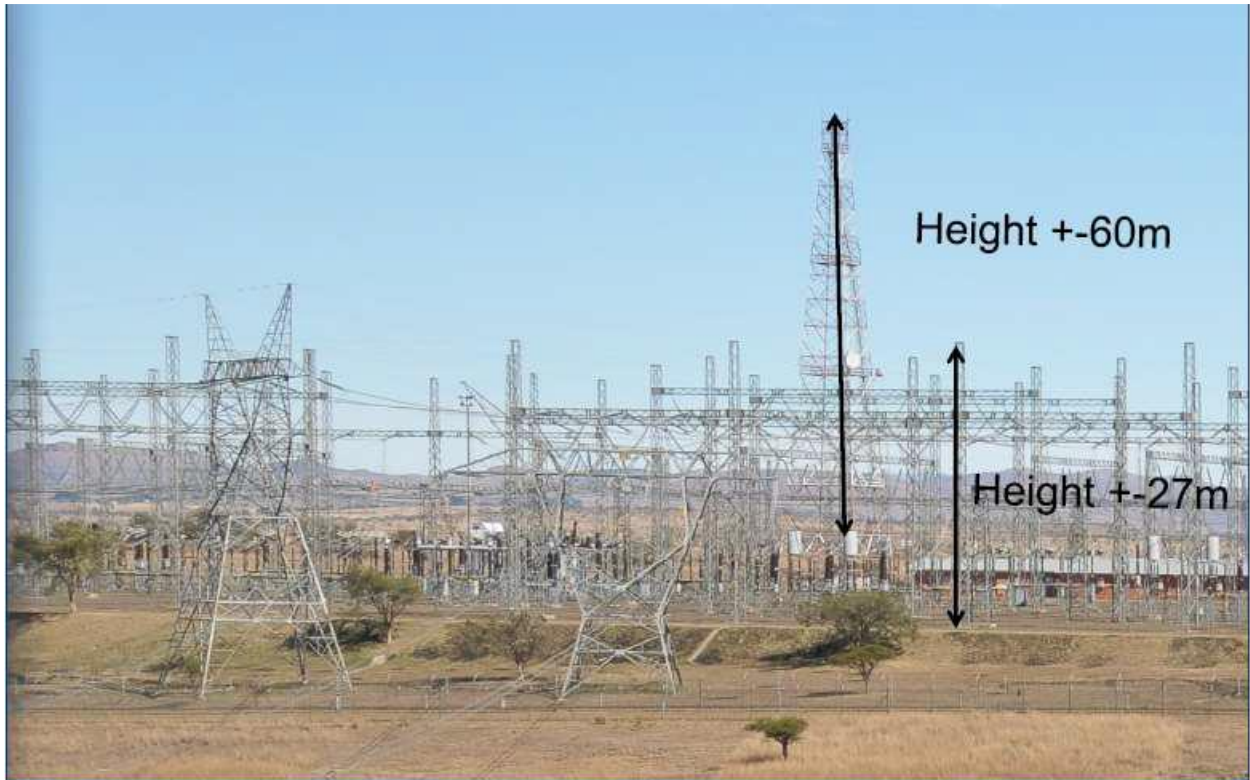
Figure 3: Side view of typical substation site
