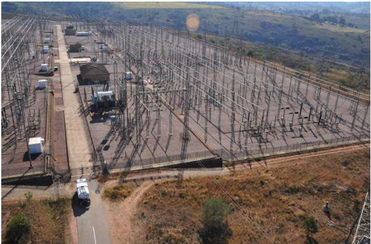
Figure 4: Typical substation site
