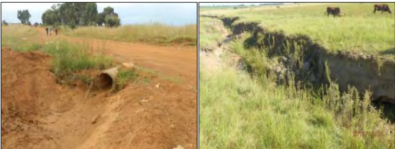
Figure 9: Photographs indicating confinement of longitudinal flow resulting in scouring and channel incision.
