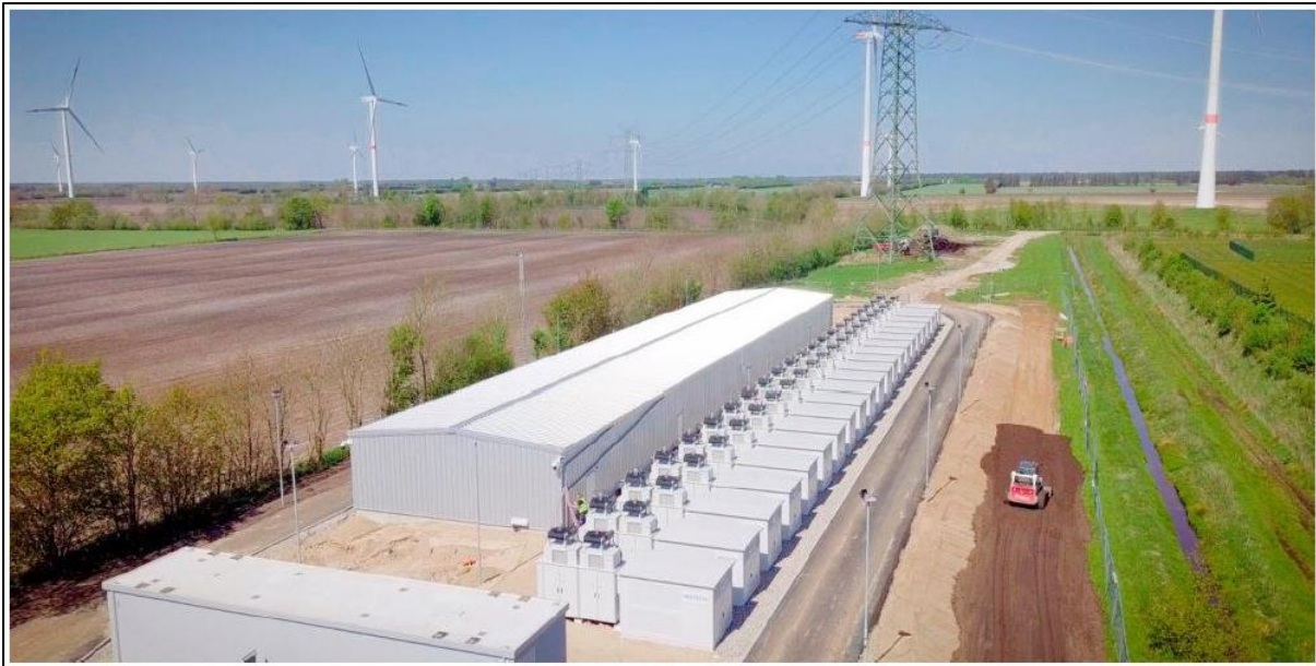
Figure 5: Typical containerized Battery Energy Storage Facility
