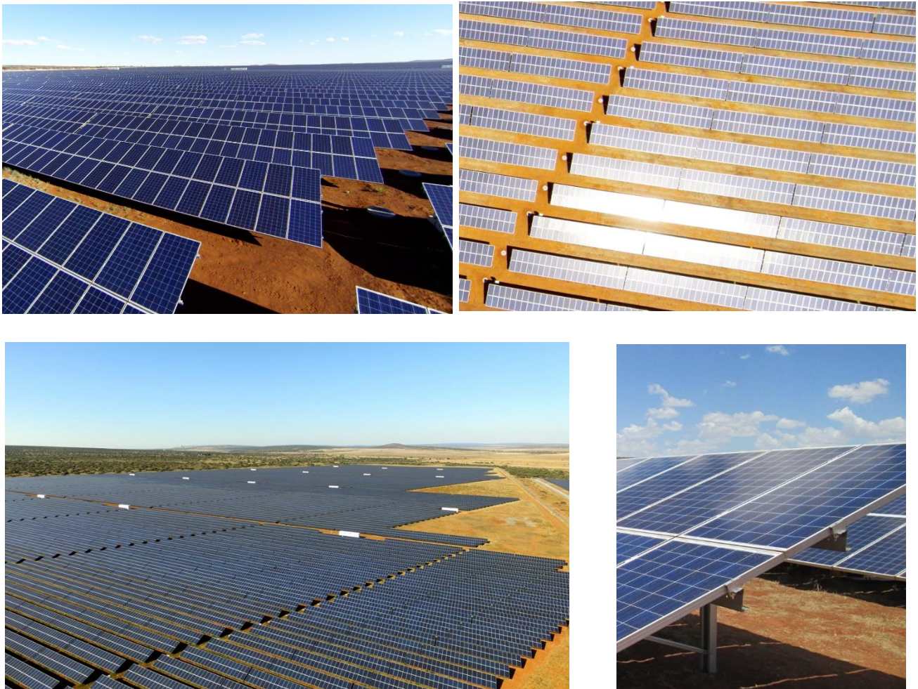
Figure 4: Photovoltaic Modules & configuration
