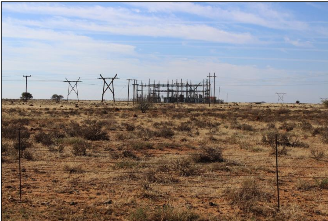
Figure 4. Jacobsdal rural substation outside Jacobsdal. Corridor 1 – Kalkaar CSP to Jacobsdal Substation (corridor approximately 19km in length)
