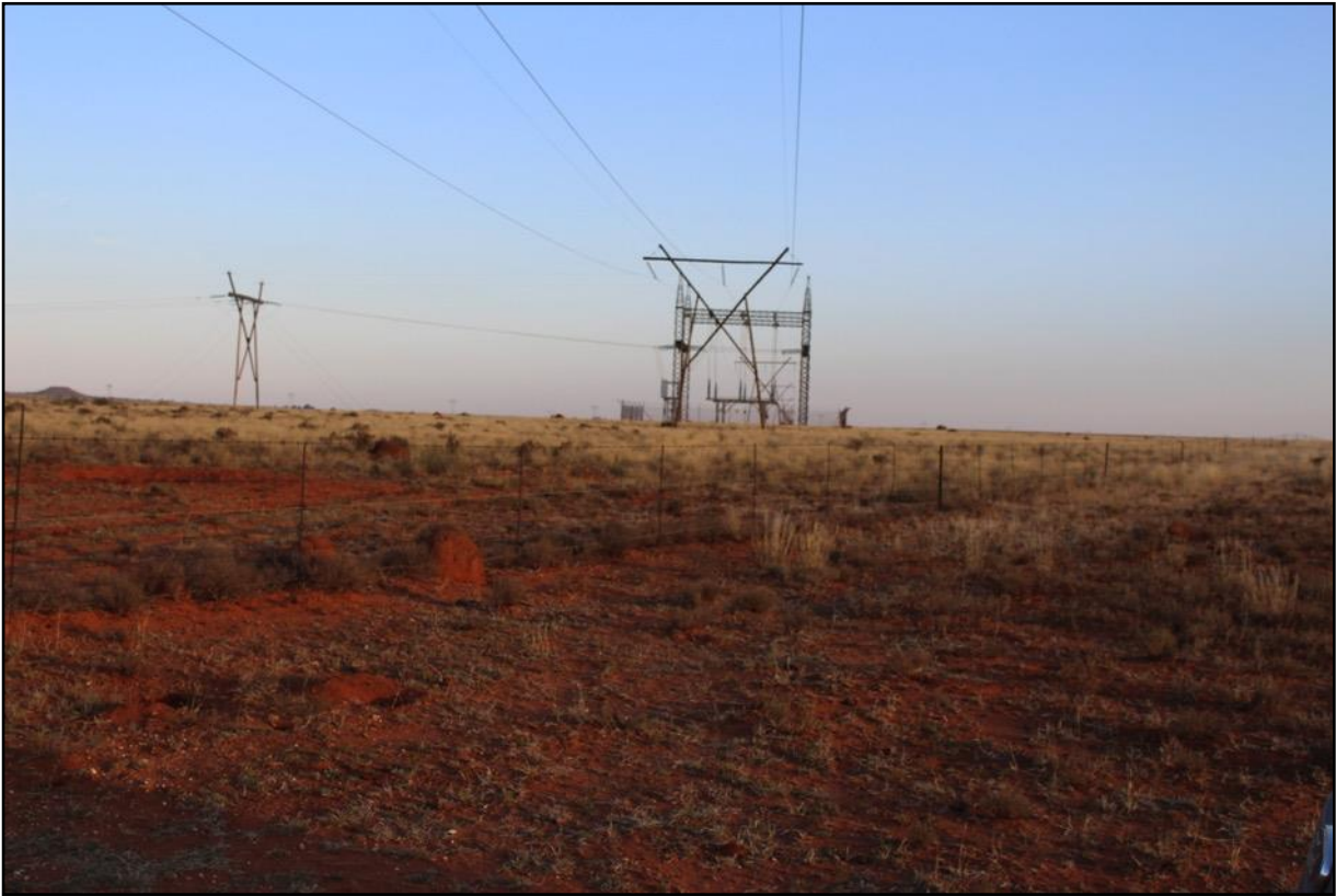
Figure 7. Skietpan switching station at the end of Corridor 1 and the beginning of Corridor 2 Alternatives 1 and 2.
