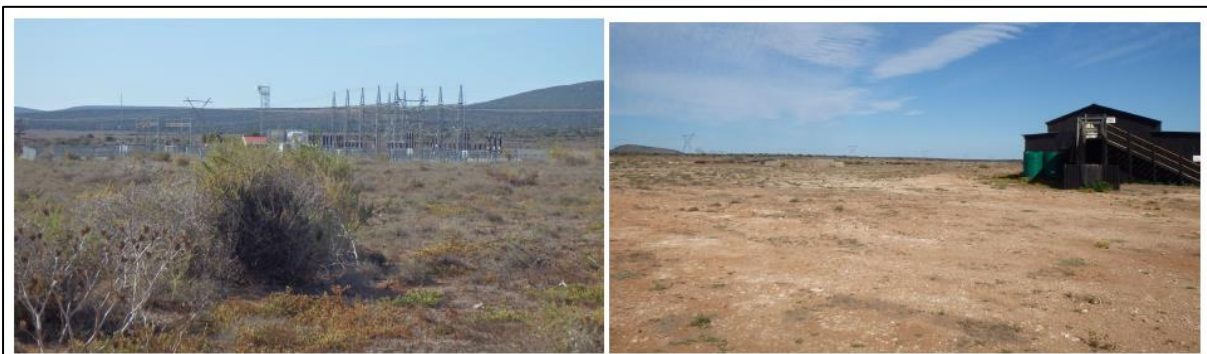
Figure 40: Skilpad substation and existing structures in the south east of the property
