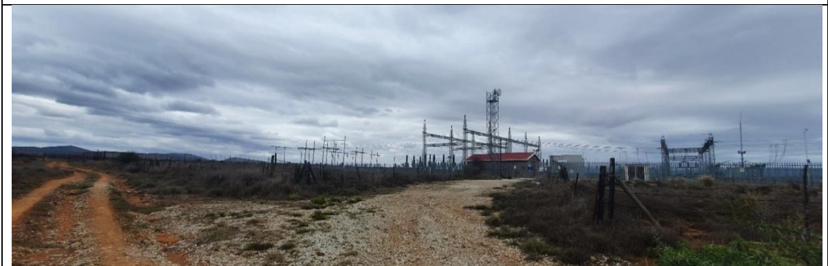
Figure 8: Existing Skilpad Substation located on the south-eastern portion of the property
