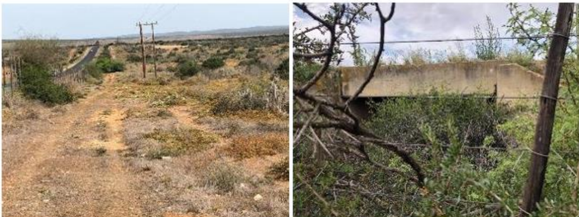
Figure 33: The vegetation of the lower reaches of the Valley with Drainage Line. Note the culvert under the tarred road.
