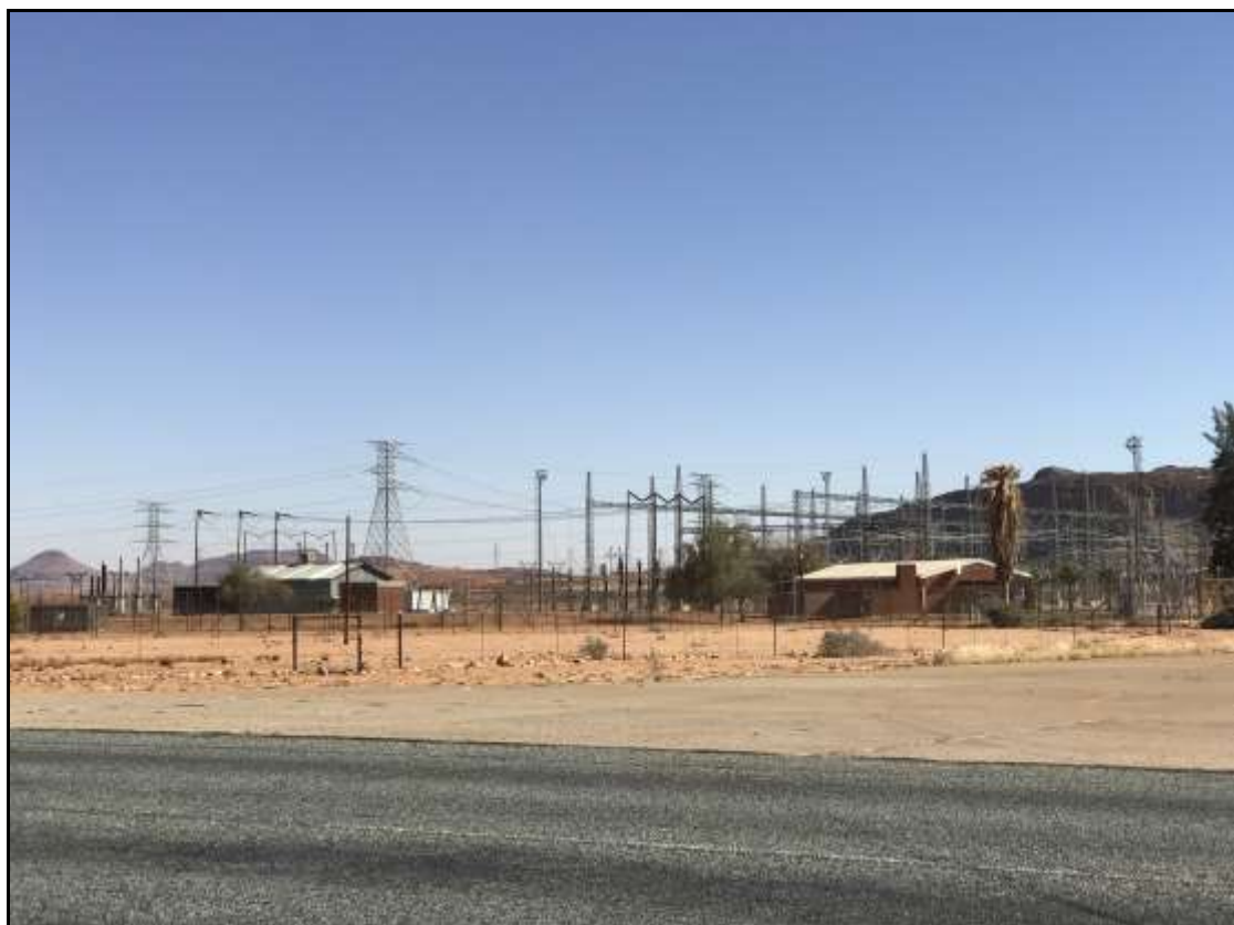
Figure 4: The Aggeneis Substation.
