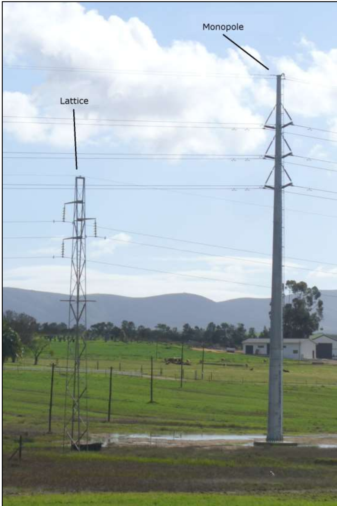
Figure 2: Conventional lattice power line tower compared to a steel monopole structure.
