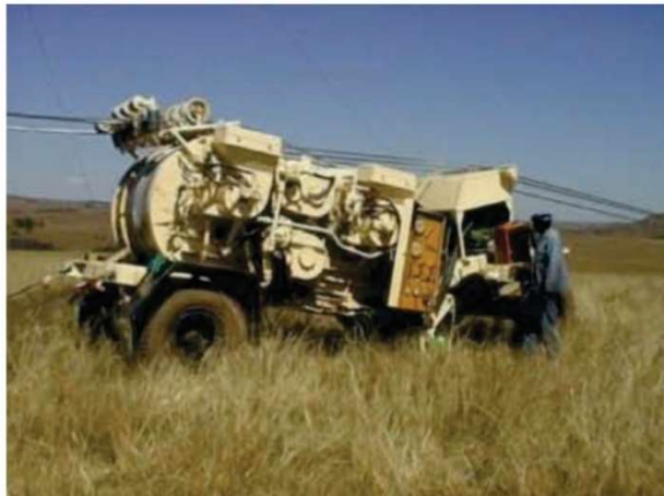
Typical example of tensioner station
