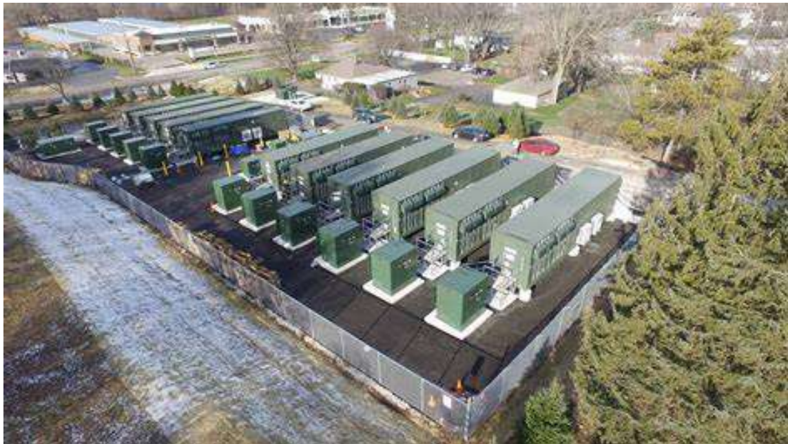
Plate 8 - Typical Battery Energy Storage System
