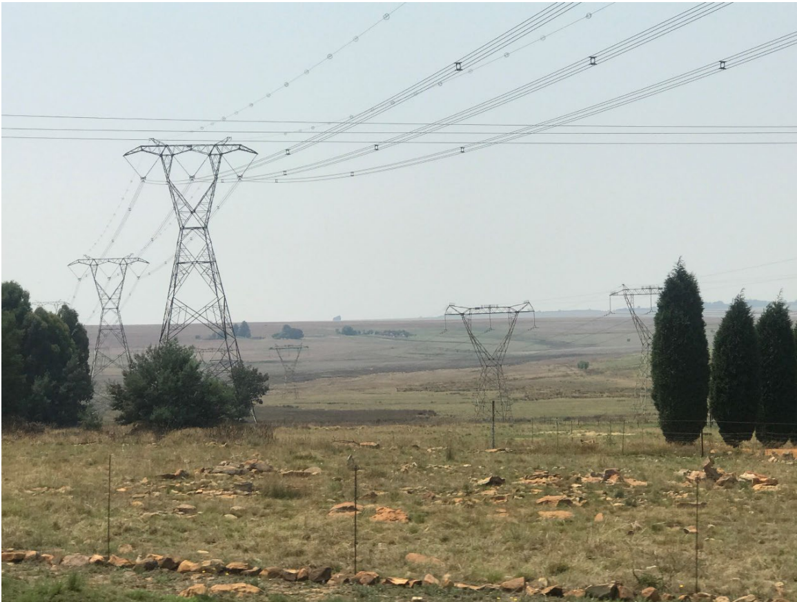
Figure 6: Existing high voltage powerlines within the study area
