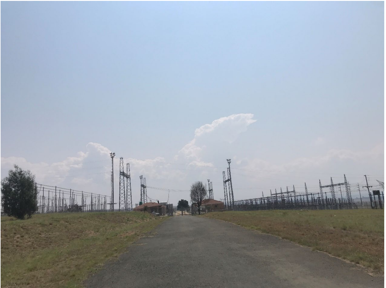
Figure 5: Existing Gumeni Substation in the east
