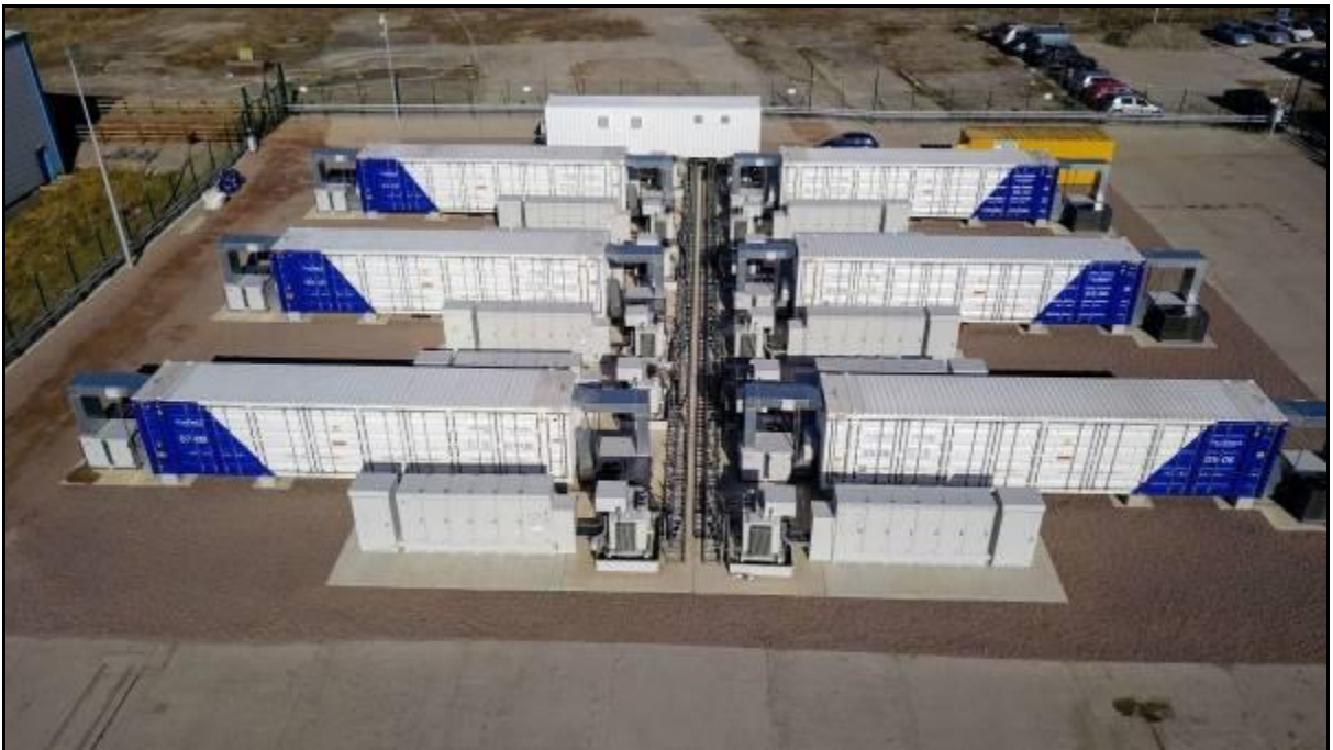
Photograph 1.2: Example of BESS located in storage containers
