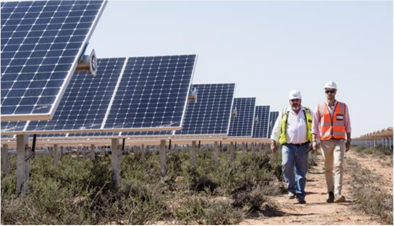
Figure 2: Photovoltaic (PV) solar panels. (Photo: SunPower Solar Power Plant- Prieska)
