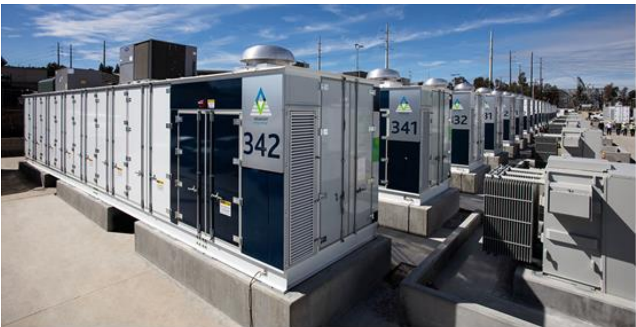
Figure 5: Close up view of a BESS (Photo: Greenbiz.com)
