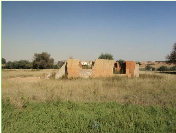
Figure 9.37: Western perspective of dilapidated building W5
