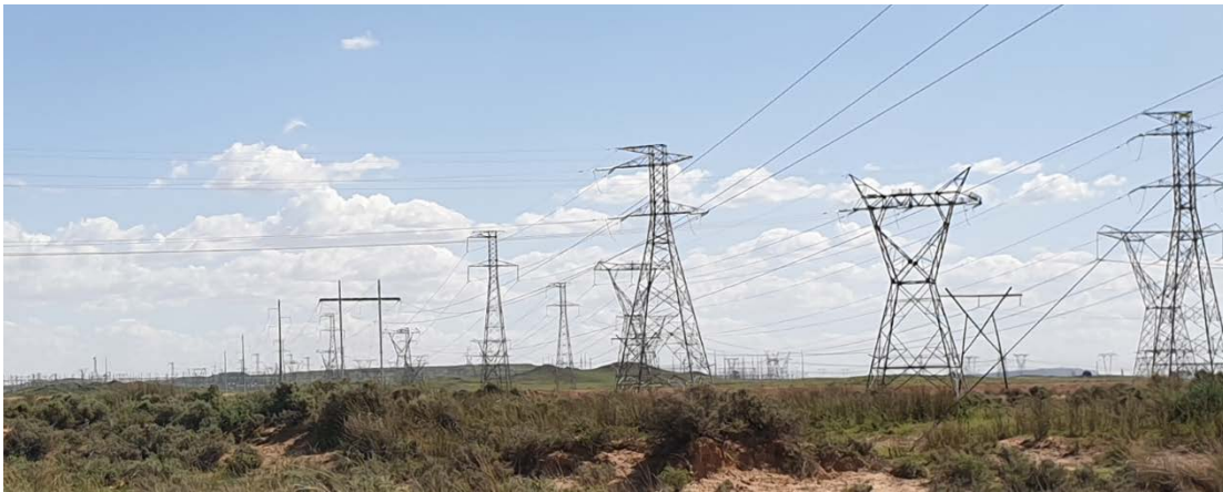
Figure 4: Multiple electricity transmission lines exist in the area, converging on the Hydra Main Transmission Substation.
