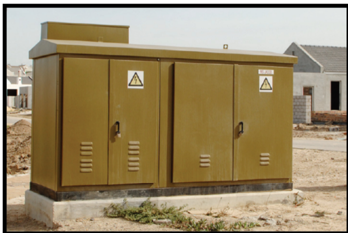
Figure 24: Outdoor distribution centre from PowerTech
