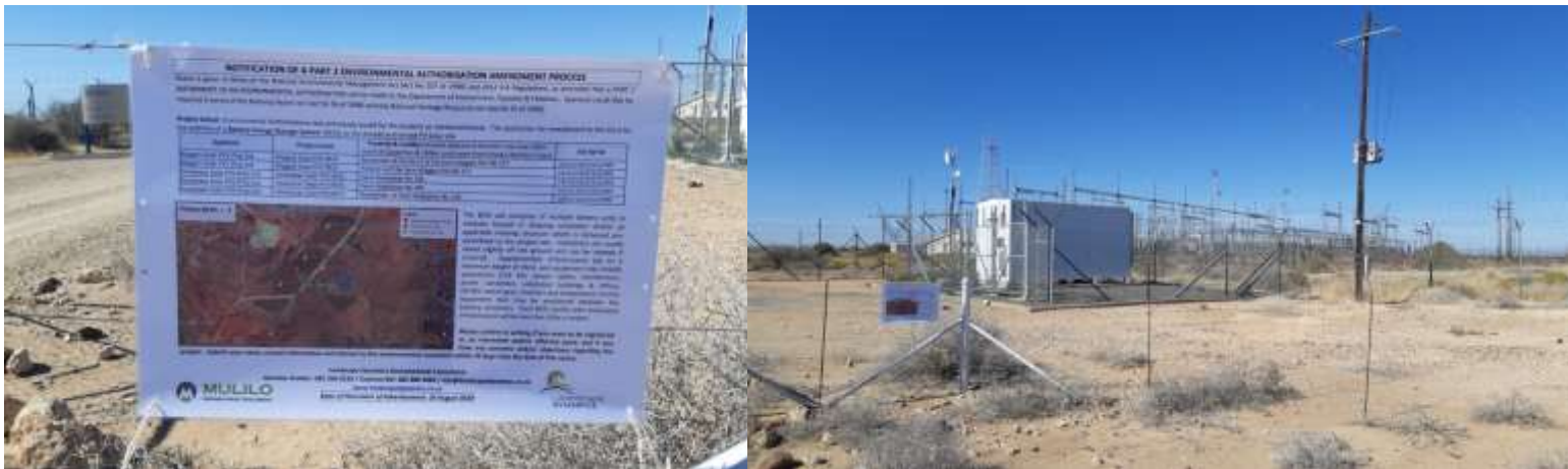
Onsite notice at the Kronos Substation
