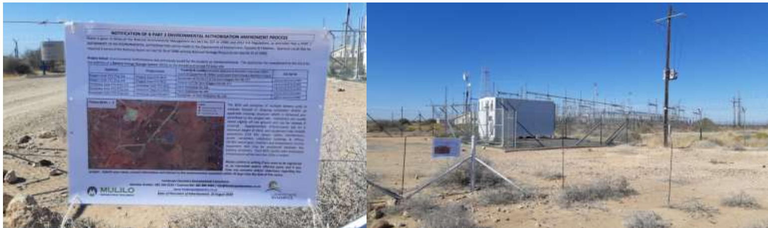
Onsite notice at the Kronos Substation
