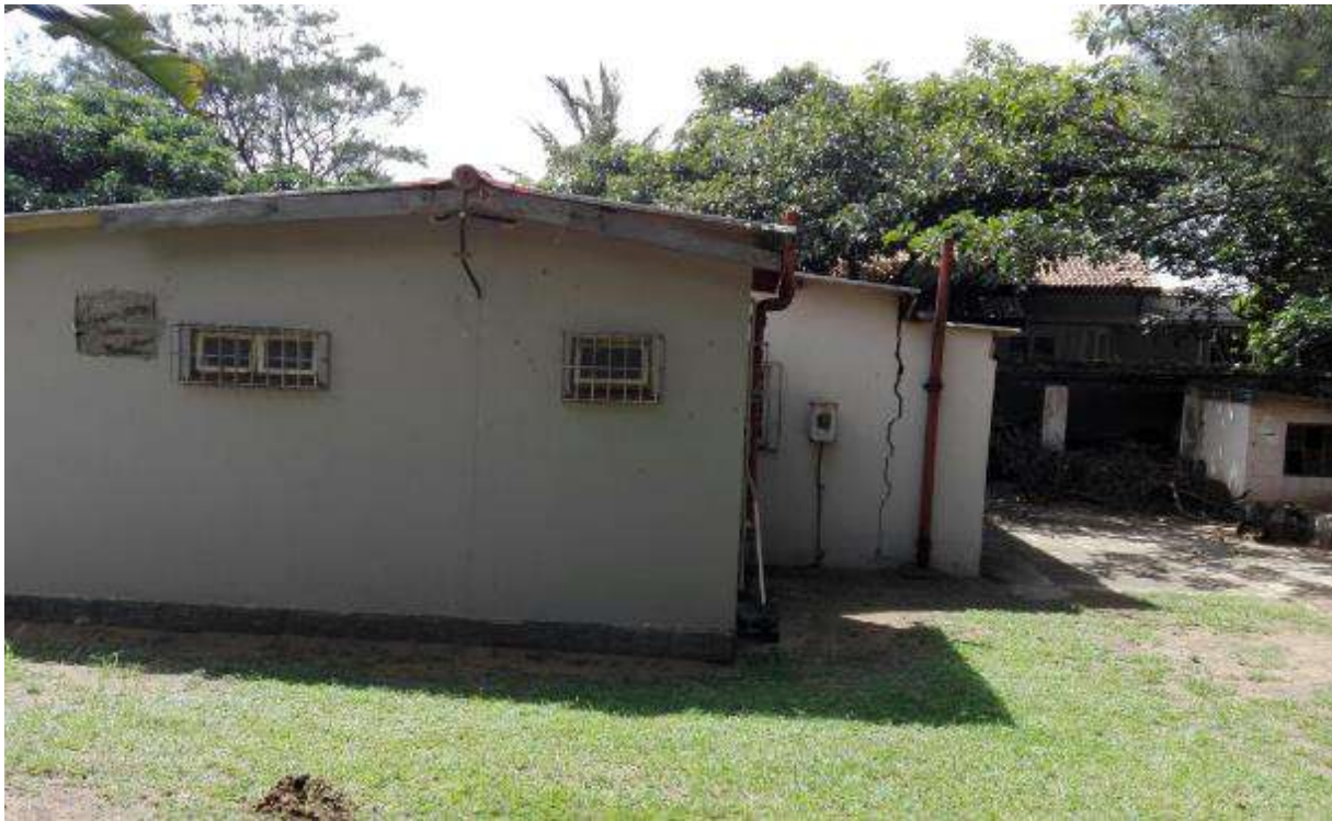
Figure 6: Side of house showing large crack
