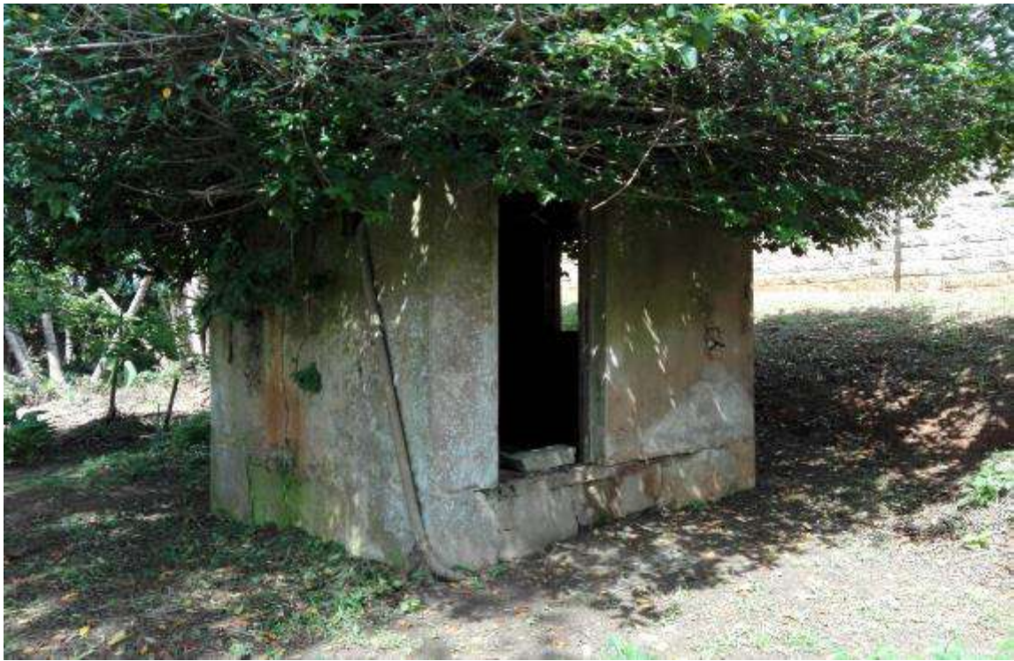
Figure 12: Old structure with tree
