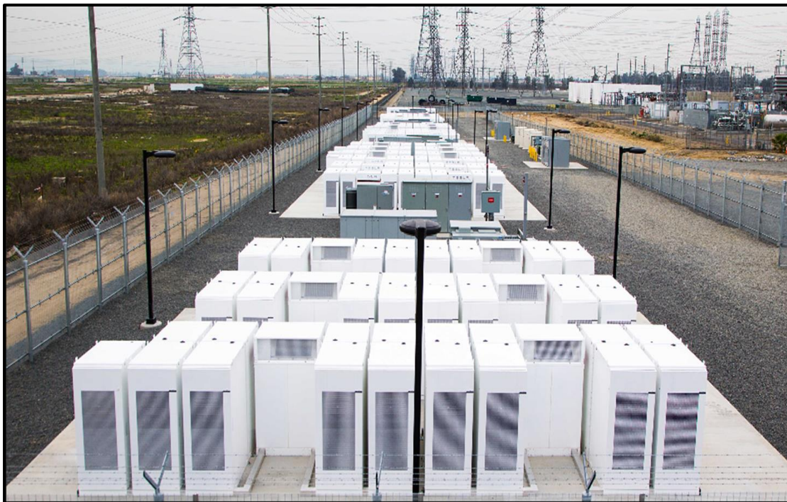
Figure 8: Solid State Batteries
