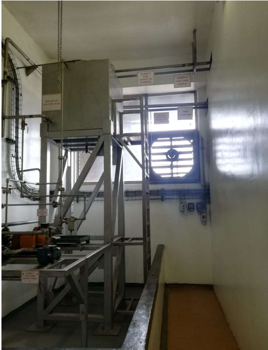
Plate 5: 1000 litre diesel day tank
