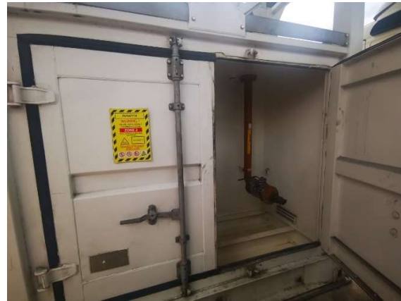
Plate 2: Opening of aboveground self-bunded paraffin storage tank
