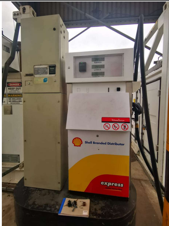
Plate 7: Fuel dispensing equipment
