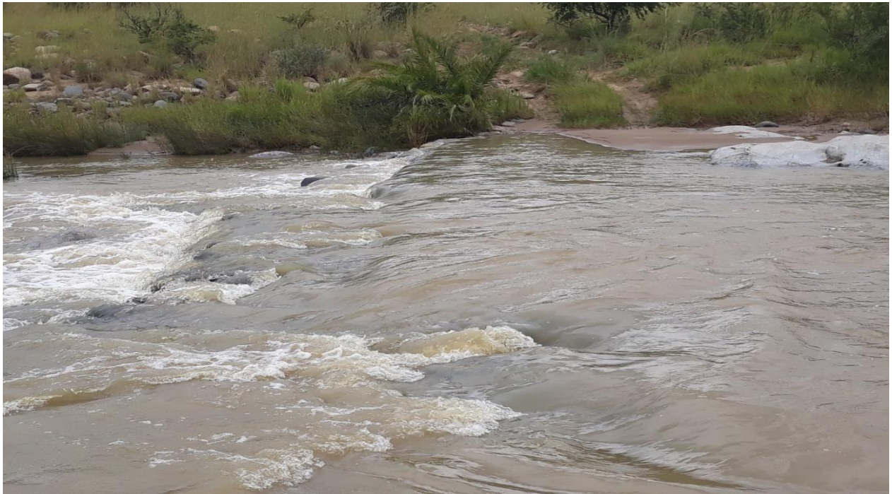
Image 2.4: Second half of the existing causeway crossing - from the North - (constantly under water)
