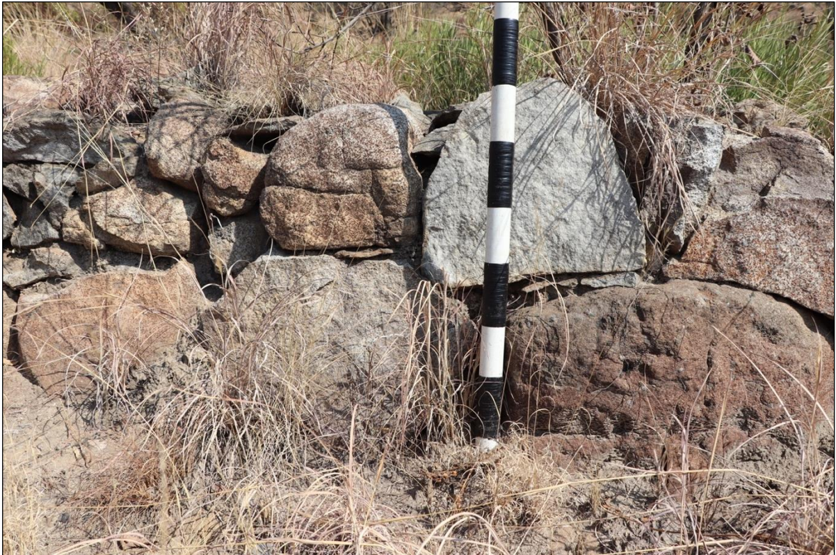
Figure 42 – Side view of a section of the enclosing stonewall. Scale in 10cm increments.
