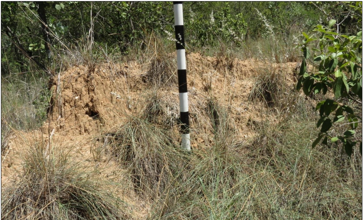
Figure 35 – This view of the smaller rectangular structure shows the height of the mud walls still remaining here. Scale is in 10cm increments.
