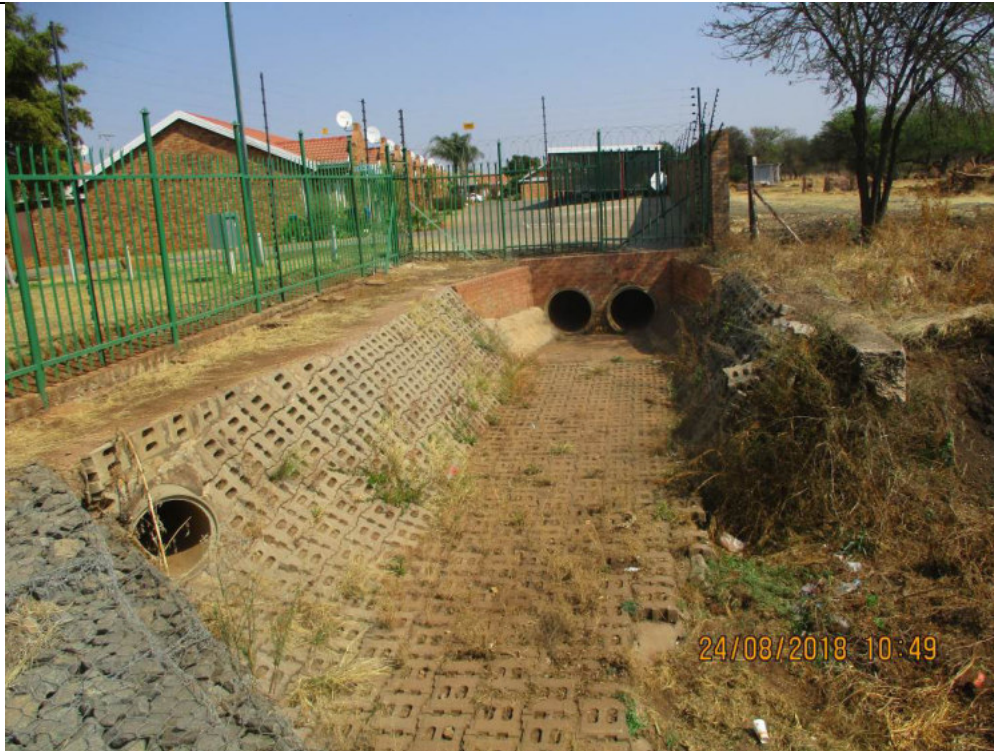
Photo 3: Existing Stormwater Pipe Outlets into Montana Spruit
