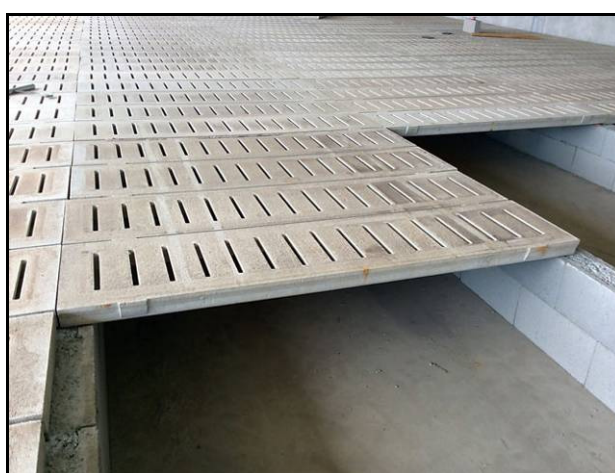
Photo 3.5: Example of the slotted floor system (obtained from www.stockyardindustries.com ).
