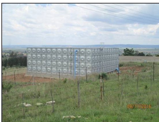
Photo 6.2: View of 2MI reservoir adjacent to the existing reservoirs at the Amsterdam WTW
