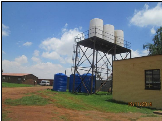
Photo 13: The JoJo tanks storing water onsite.
