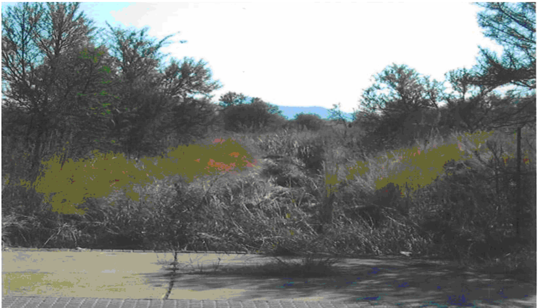
Photo 2.7.3: Thick overgrown from pipe culvert downstream at Tsamma Road
