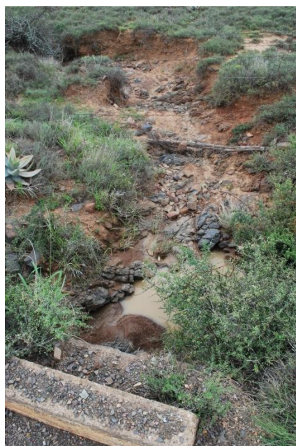
Plate 6: A water course crossing with no downstream erosion protection that has lead to river bank scour and channel incision
