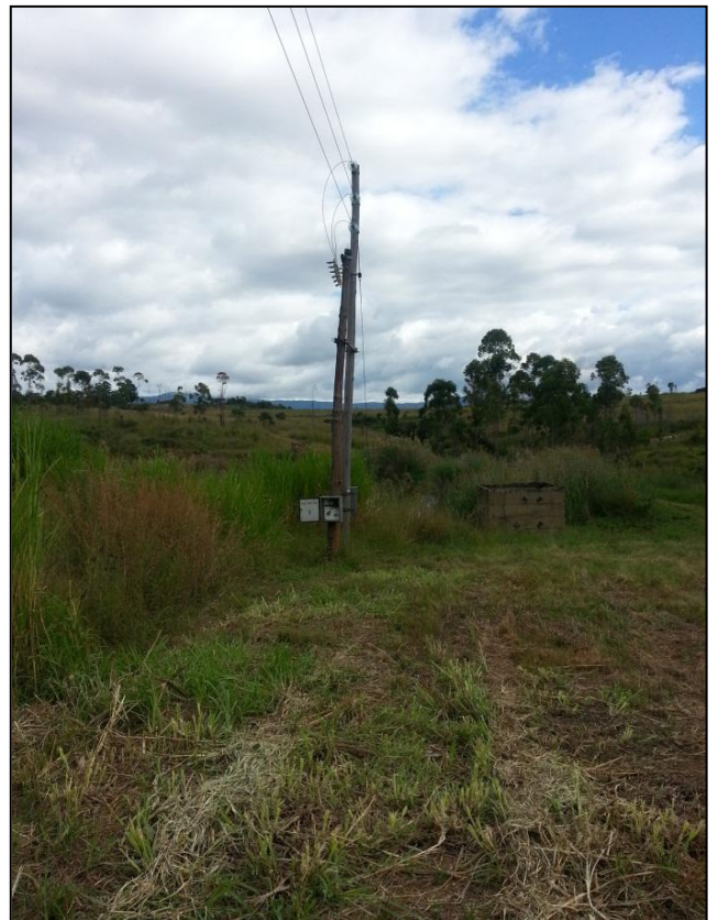
The Eskom electrical pole for the pump station at the dam
