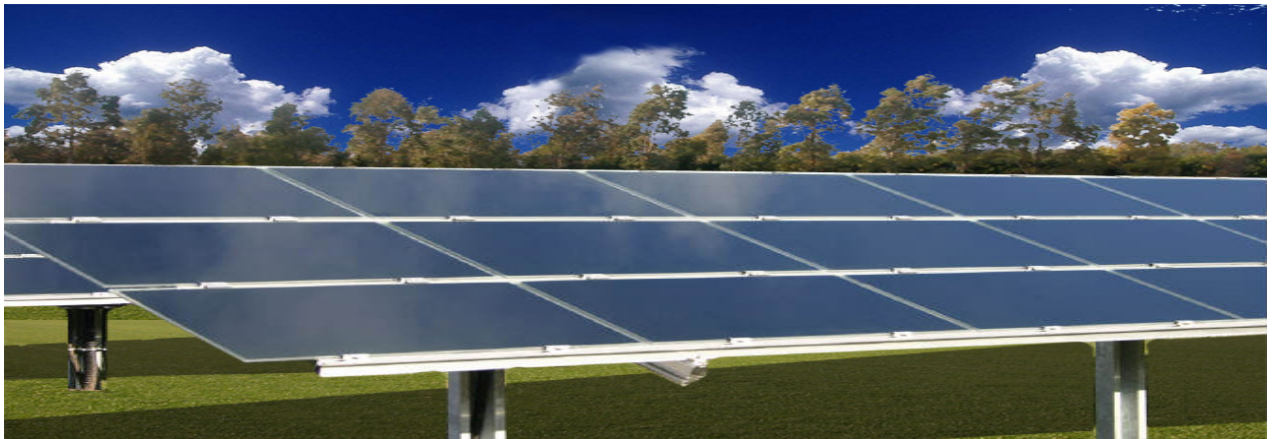
Figure 4 Frontal view of PV arrays mounted on fixed mounting systems
