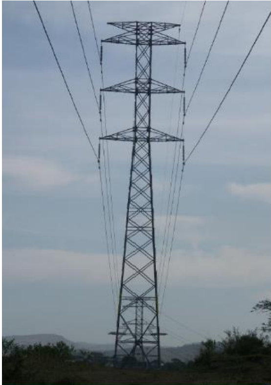
Plate 1: 245A double circuit suspension tower
