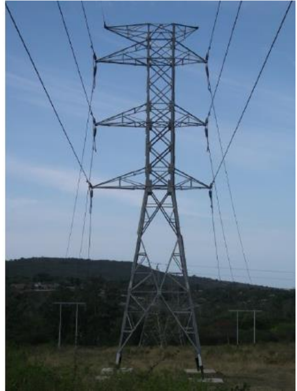
Plate 2: 245D Angle Strain Tower
