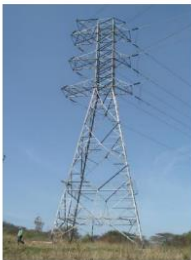
Plate 3: 245E Terminal Tower
