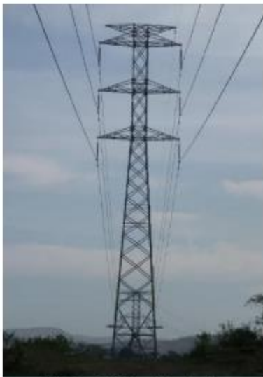
Plate 1: 245A double circuit suspension tower
