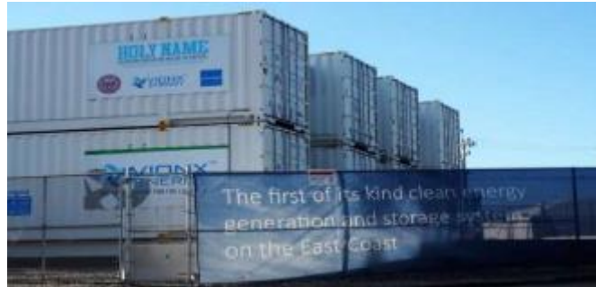
Source – Bushveld Minerals and Energy – Energy Storage and Vanadium Redox Flow batteries 101 – 13 November 2018.
