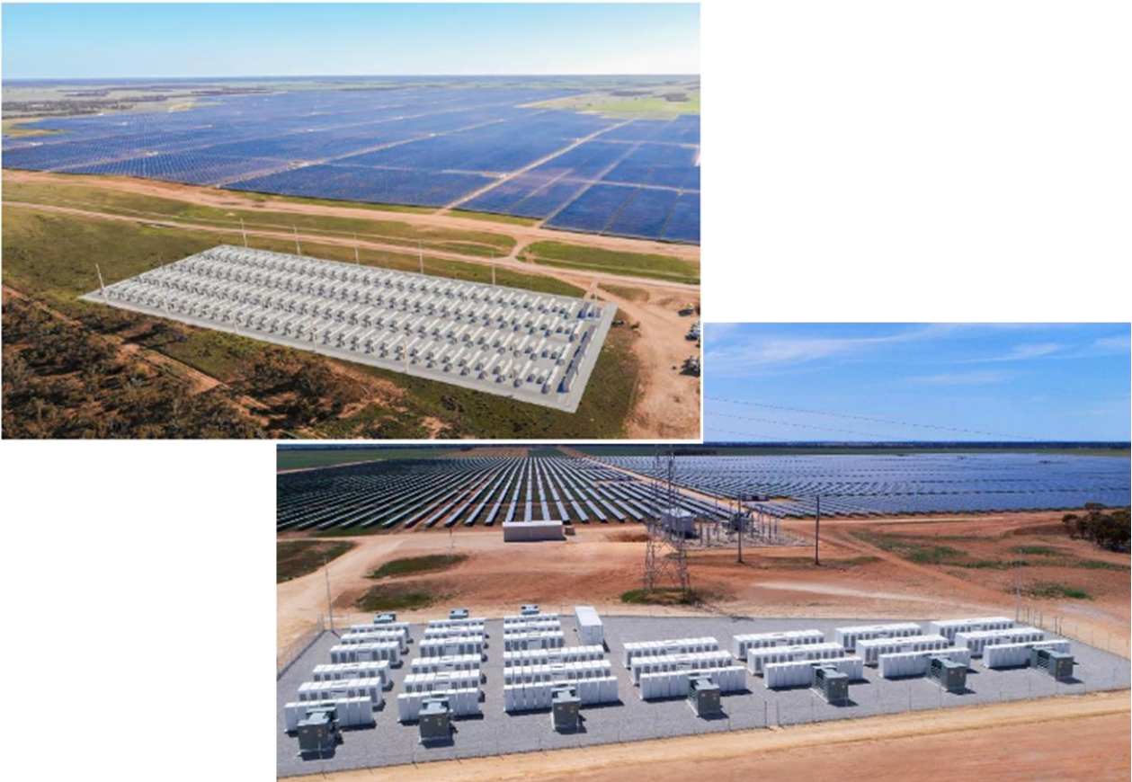
FIGURE 2.3.2.1 – Images of Typical BESS Systems Servicing Solar Power Farms
