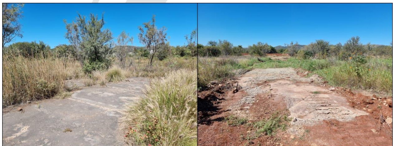
Figure 69: View of a Building Floor And Foundation Structure In The Project Area at TWRD-FT01.
