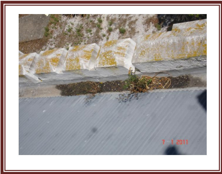
Fig.9.6 Blocked box gutter.
