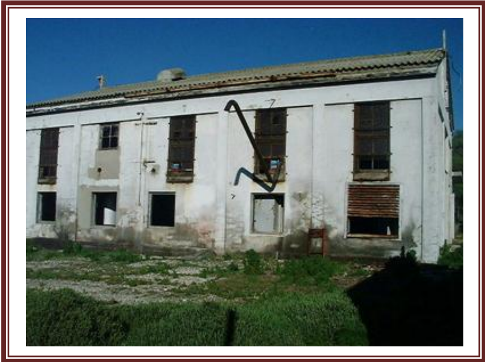
East elevation main building ca 1996. Note fire bucket stand and grill opening in section E
