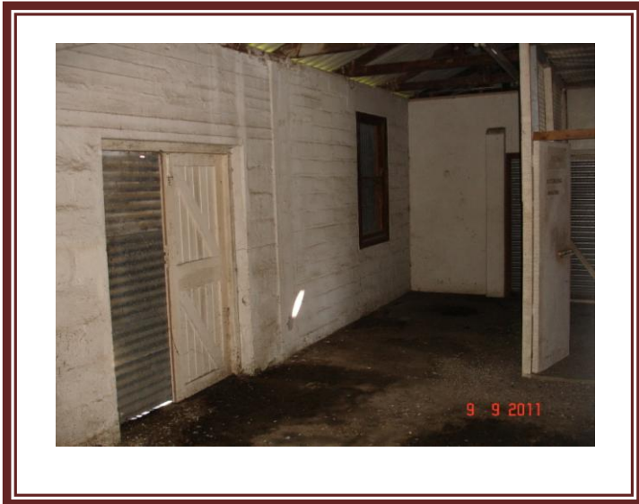
Fig.38. Interior of door boarded up
