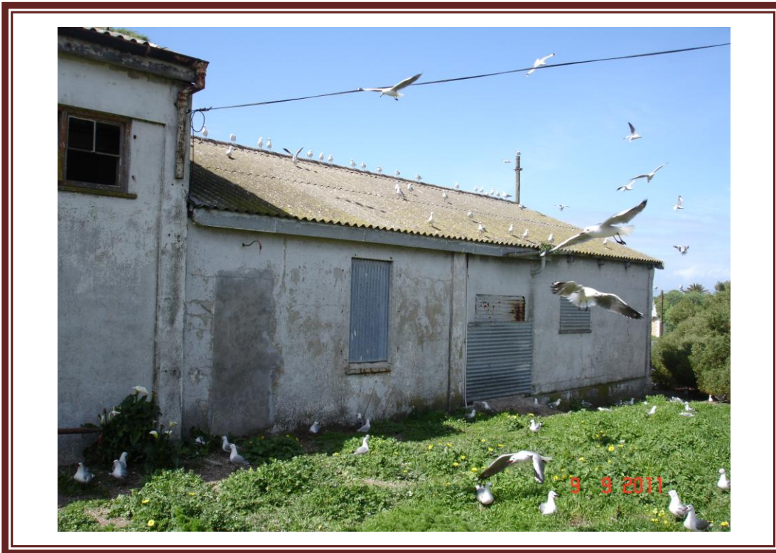
Fig. 55. Remainder of gutter and downpipe west face Extension.
