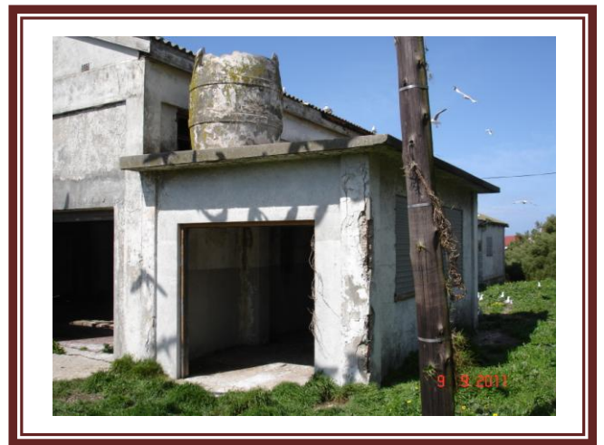
Fig.32. Right, tank on roof of transformer room
