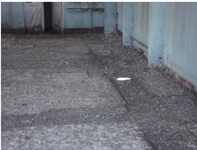
Fig.23. Showing skirting outline with missing tiles.
