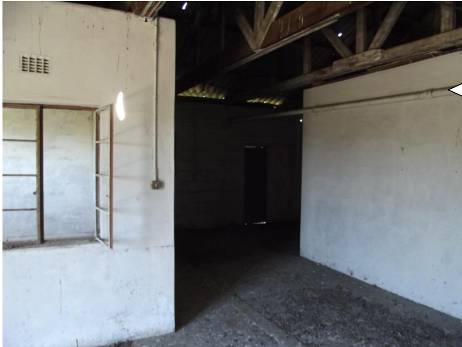
Fig.23. Steel rain water pipe through building.
