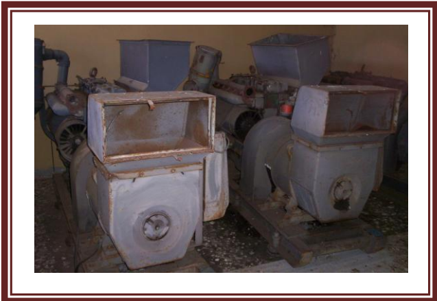
Fig. 14. Lister diesel gensets ca 1968
