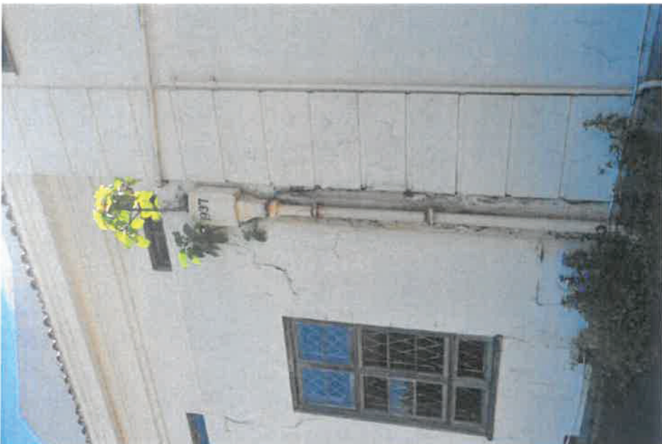
CAST IRON DOWNPIPE, 1937 to hopper+head, with vegetation.
